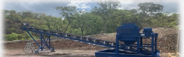
Upgraded Crushing Circuit
